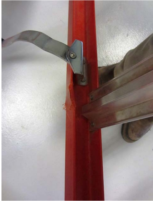
Photo 2 Bend ladder brace
